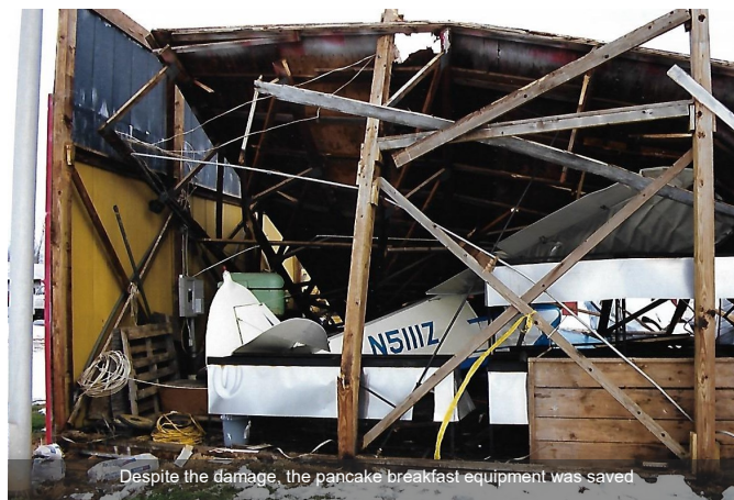
A Piper Warrior inside the collapsed hangar.
