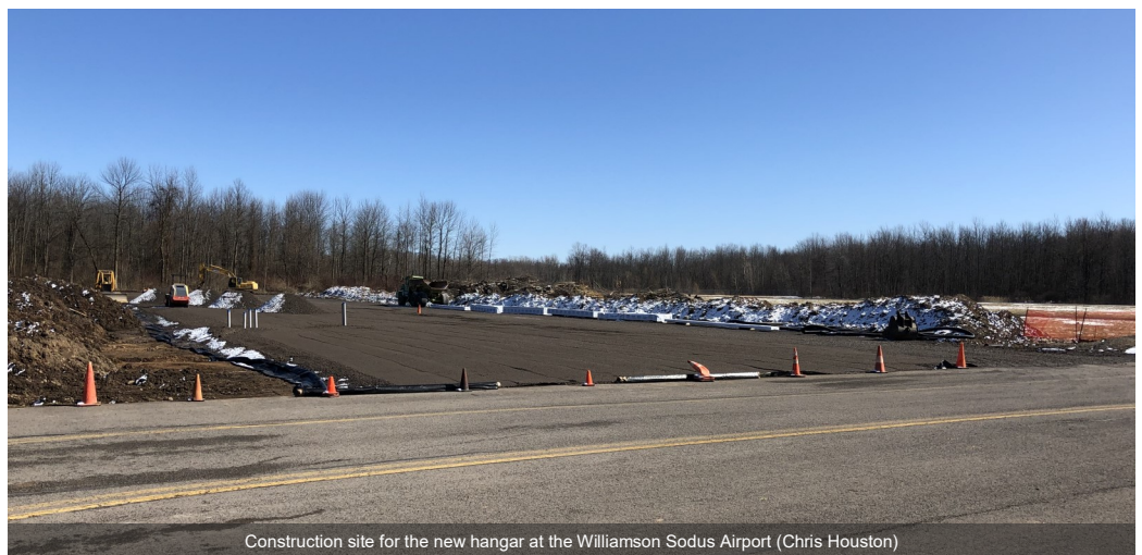
Construction site for the new hangar at the Williamson Sodus Airport (Chris Houston)
